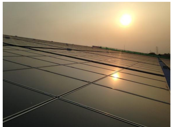
Solar PV system, Credit: Solventia Solar in Thailand
