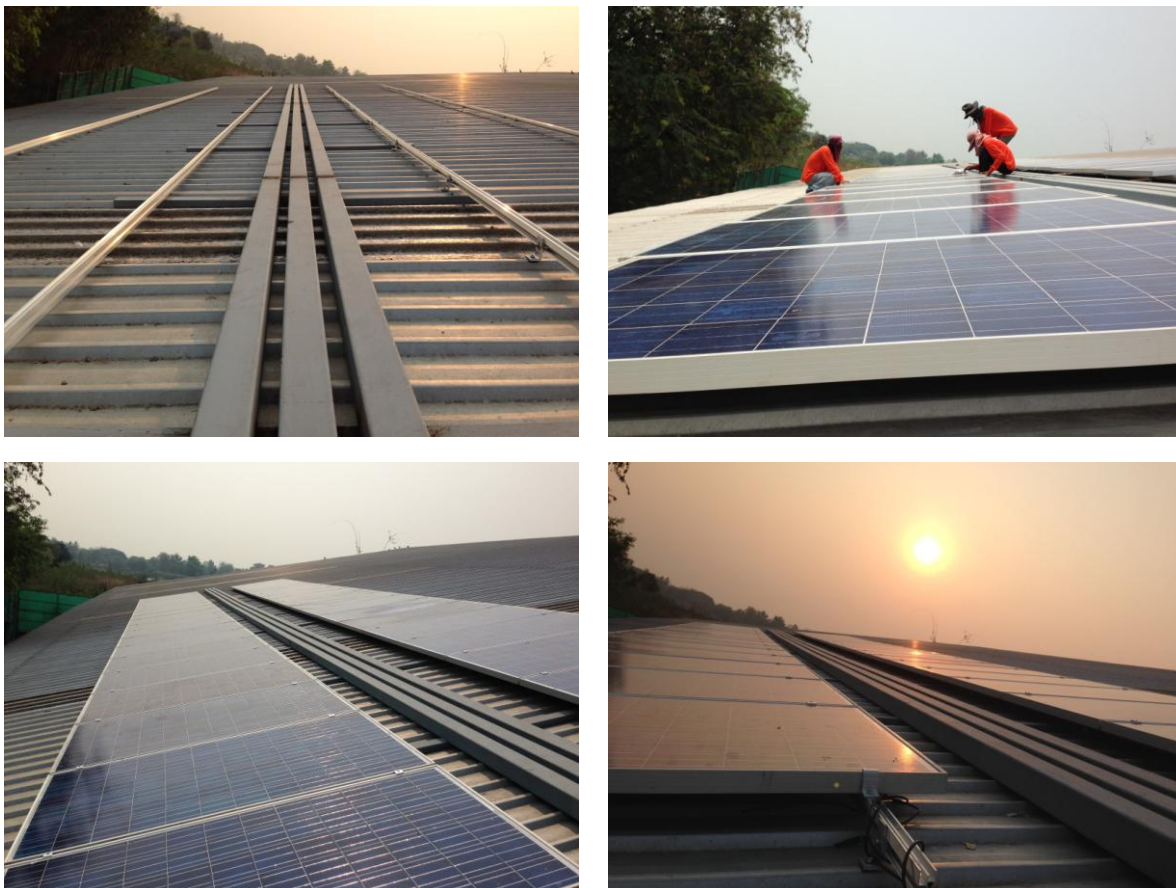
10 kWp Solar PV System at Sri Thana Rice Mills, Credit: VE Solar
