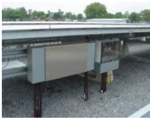
Collection & Combiner boxes
