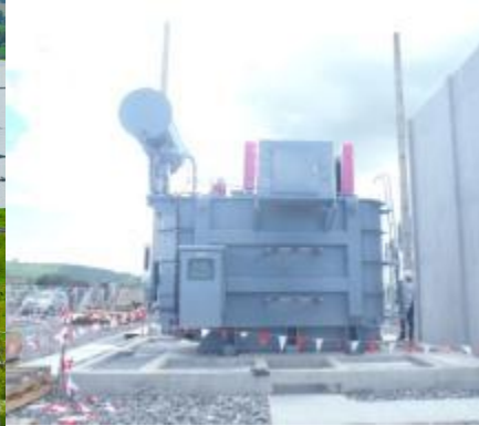
22/115kV Power Transformer
