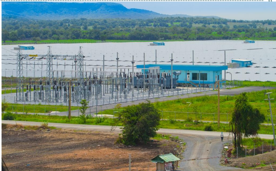
- 115kV Switchgear & 115kV NED Substation
